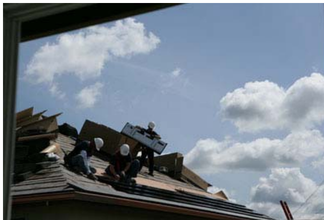
Workmen install PowerLight panels on the model homes of the new Avignon community by Centex Homes in Pleasanton. (Photo courtesy of Centex Homes)
